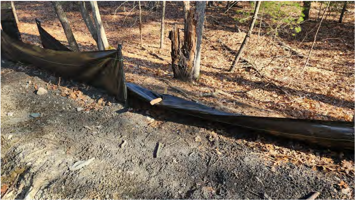
Photo 8: Broken stake in the silt fence along segment 8. Photo taken on 3/30/23
