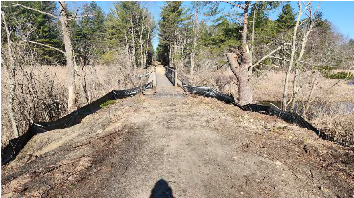
Photo 9: Silt fence functioning properly at Hop Brook Bridge along segment 7. Photo taken on 3/30/23
