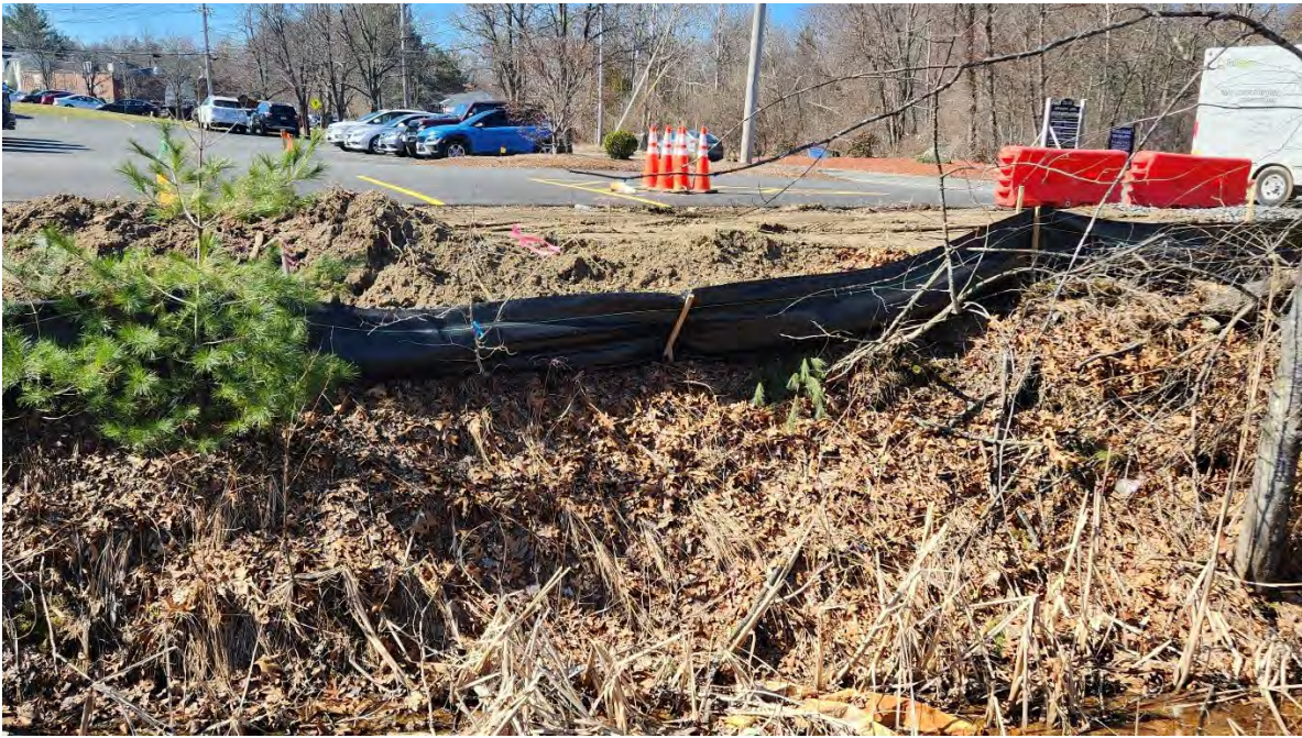
Photo 4: Broken silt fence stake and notable sagging in the fence along segment 12. Photo taken on 3/30/23
