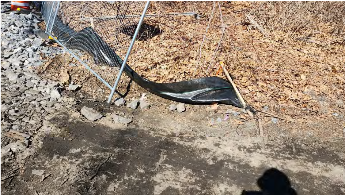
Photo 2: Broken silt fence stake that needs to be replaced at construction entrance (SUB STATION).
