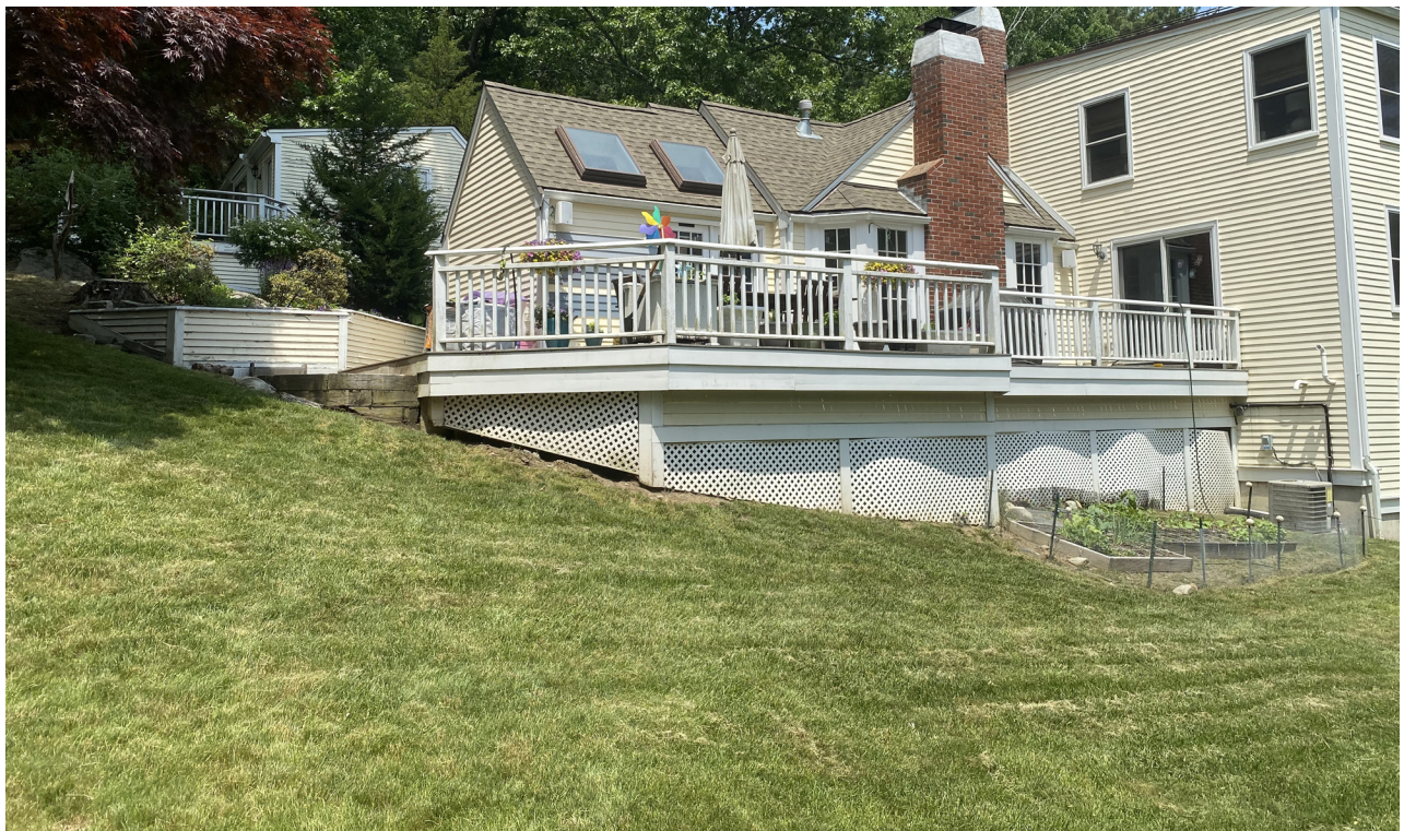
REAR DECK & WESTERN SLOPE. AREA FOR PROPOSED STEPS & WALK (SOUTH WEST) - SPRING 2022
