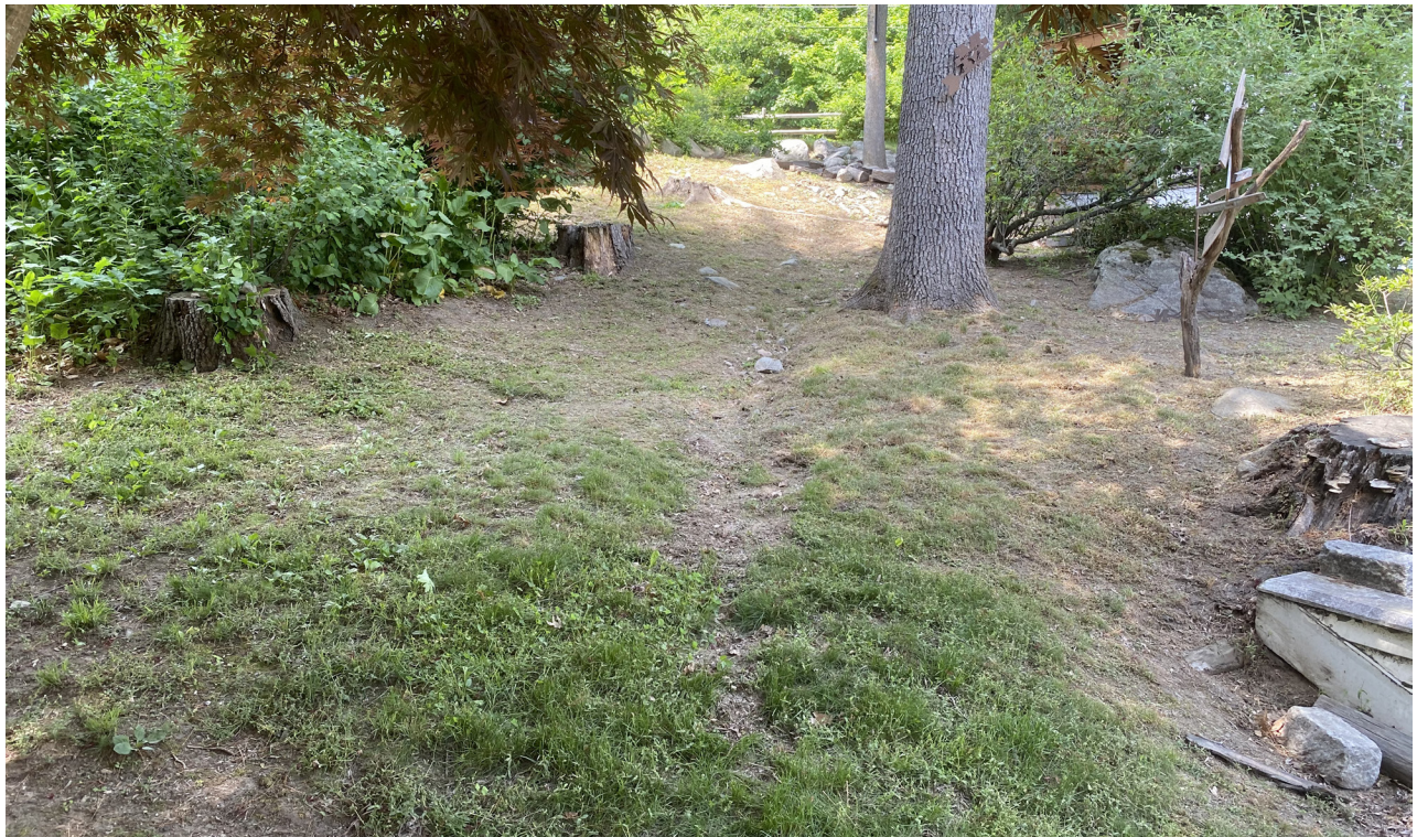
EROSION ON WESTERN SLOPE. AREA FOR WATER RETENTION (WEST) - SPRING 2022
