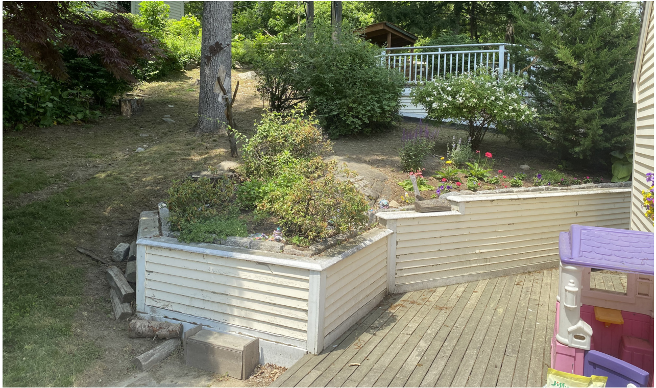
TIMBER WALL & ERODING WESTERN SLOPE (WEST) - SPRING 2022
