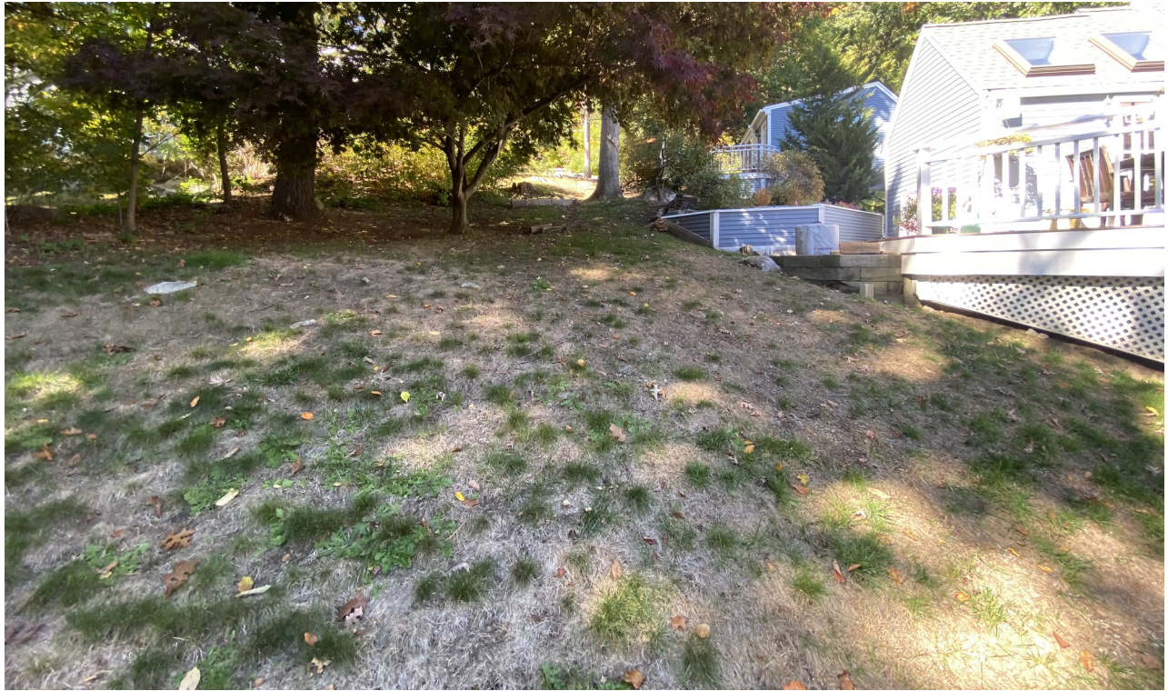
WESTERN SLOPE EROSION. AREA FOR PROPOSED STEPS (SOUTH WEST) - FALL 2022
