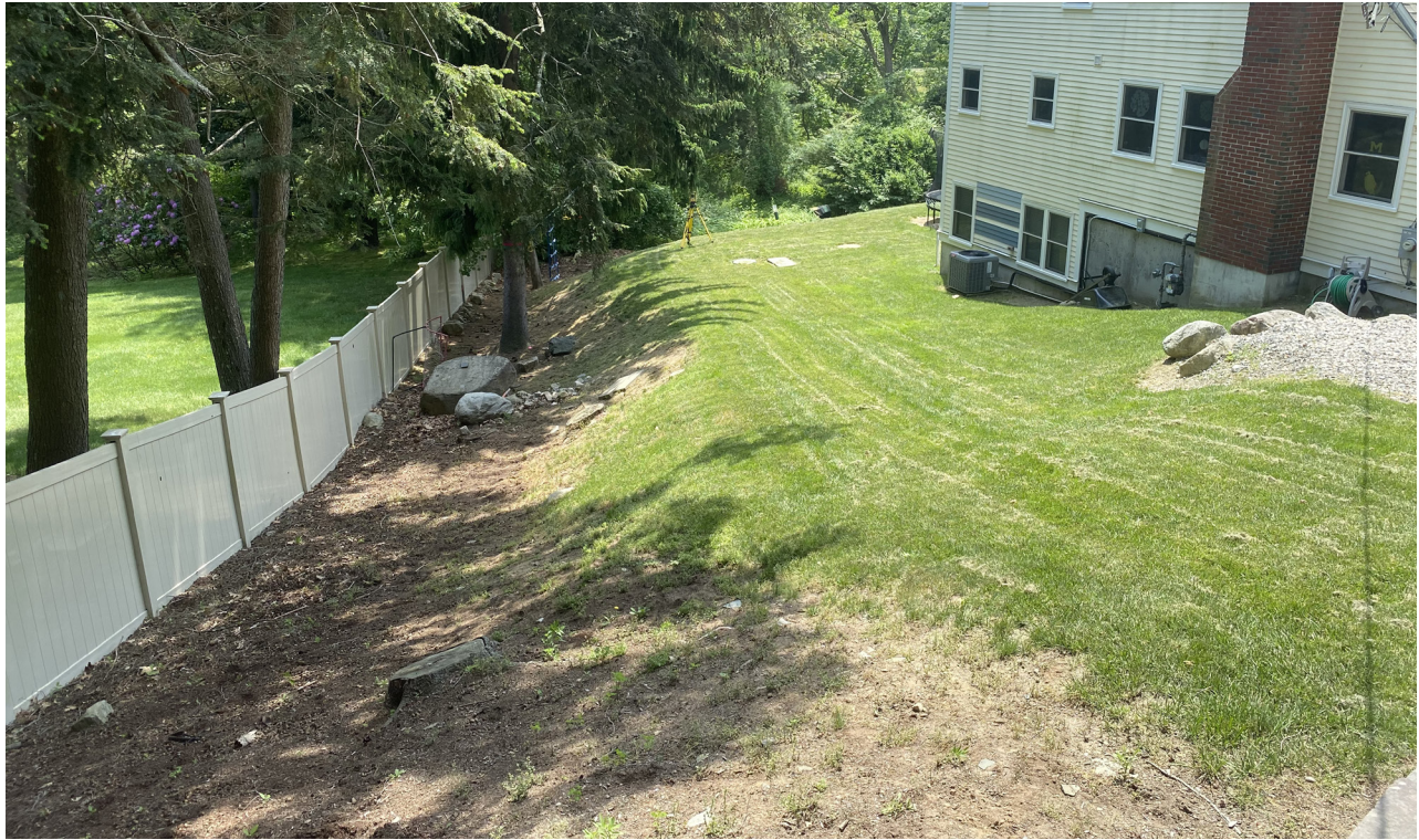
EASTERN LAWN AND ERODING SLOPE LOOKING SOUTH (NORTH EAST) - SPRING 2022
