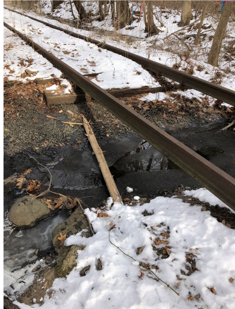
Photo 2. Overview of railroad tracks over tributary to Hop Brook within proposed work area at Culvert 4
