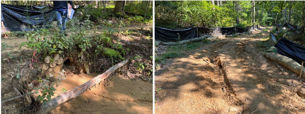
Section of White Ridge Trail that needs sediment removal. Photo taken 9/9/22.
