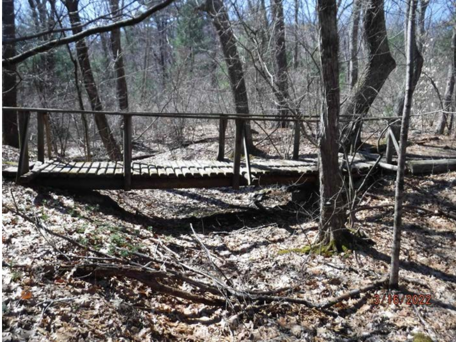
Photograph 51: Existing bridge crossing of Intermittent Stream 11 (Little Sachem Brook)/Wetland L; bridge to be replaced with wood platform bridge.
