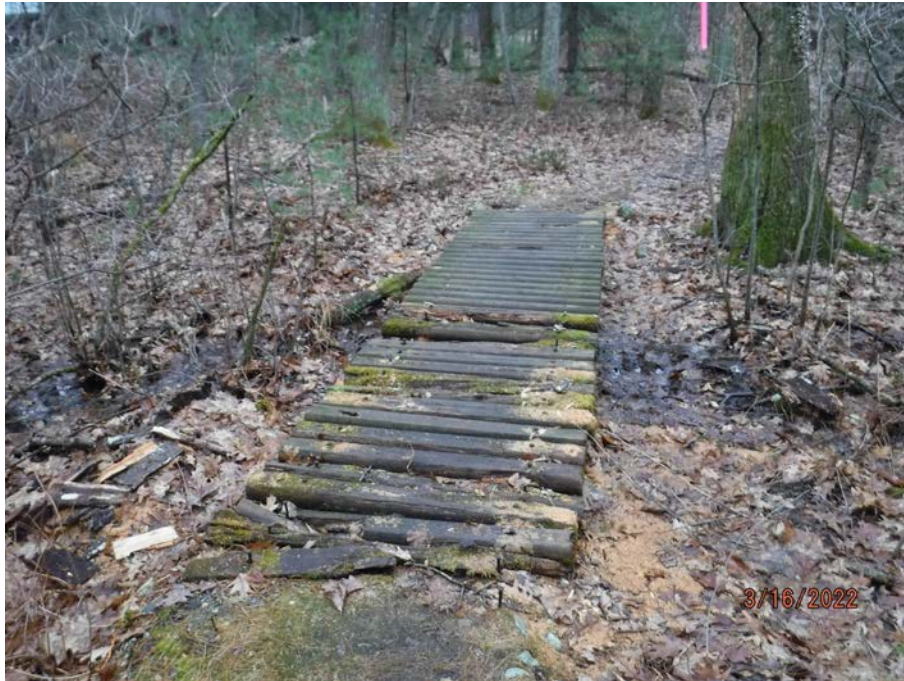
Photograph 47: Existing crossing of Wetland E, wood timber footbridge near WFE-422 to be replaced with wood platform 'bog bridge' on concrete piers.
