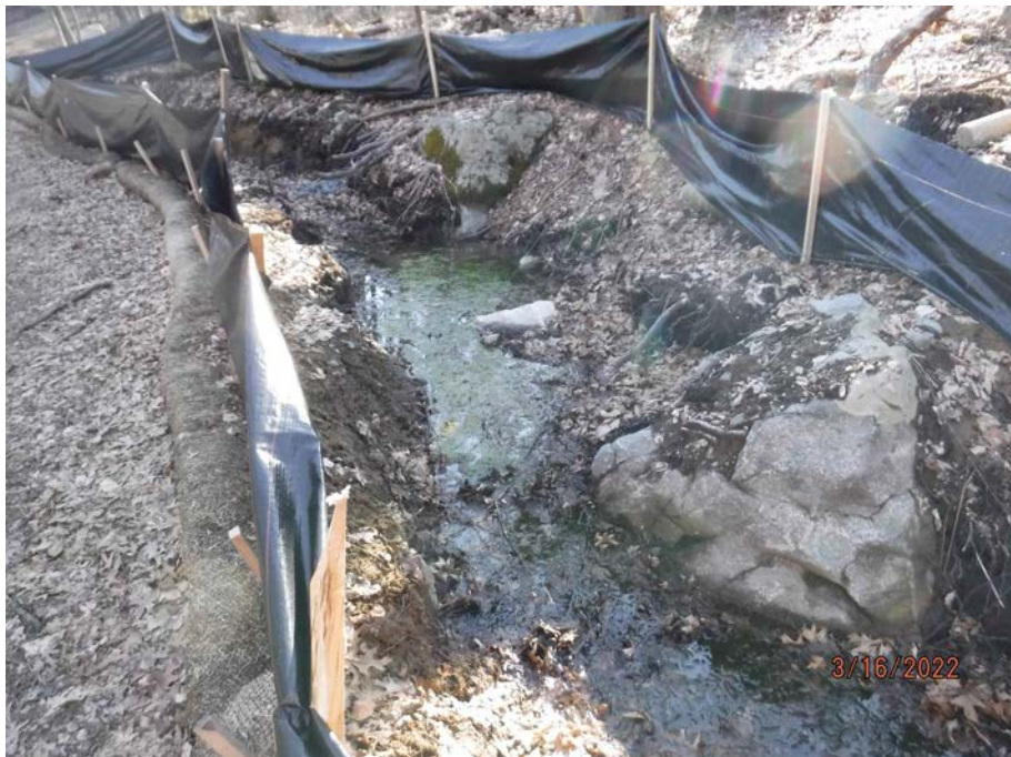
Photograph 54: Upgradient swale (typical) that flows to Wetland M to be stabilized with check dams, loam, seed, and biodegradable erosion control straw matting.
