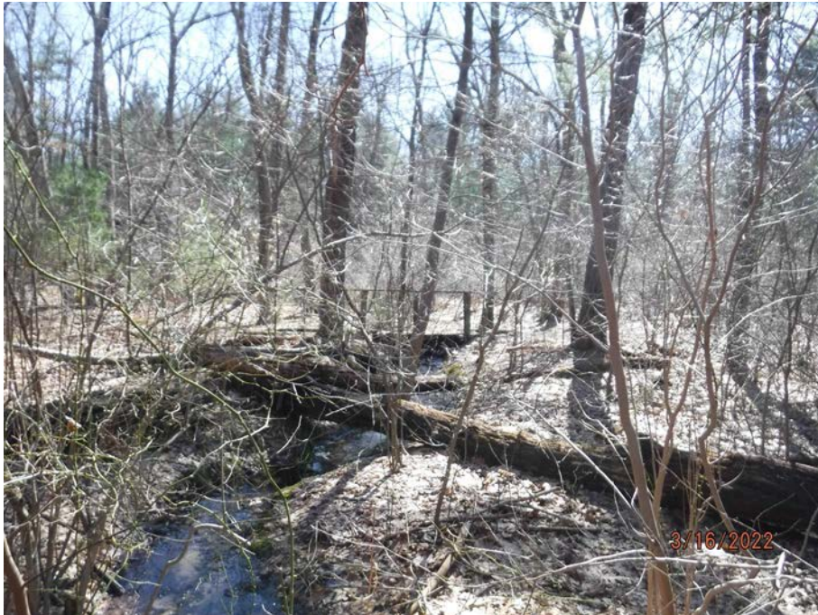
Photograph 52: Existing bridge crossing of Intermittent Stream 12 (Big Sachem Brook)/Wetland L; bridge to be replaced with wooden platform bridge.
