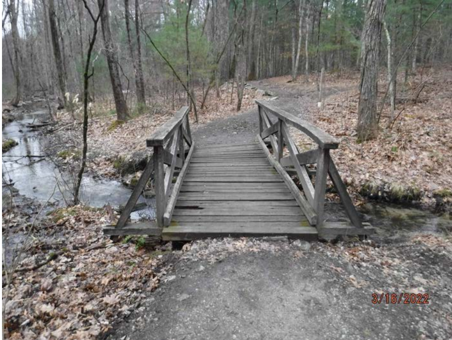
Photograph 49: Existing wooden crossing in disrepair at Stream 10/Wetland K; bridge to be replaced with wood platform bridge on reinforced concrete footings.
