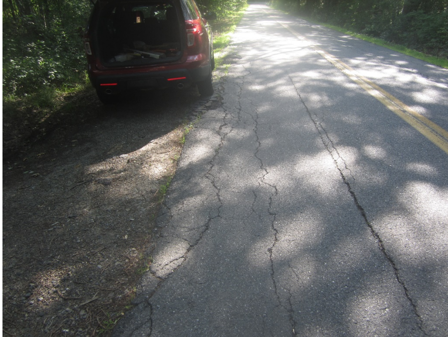
Picture 1: Area requiring full-depth repair.
