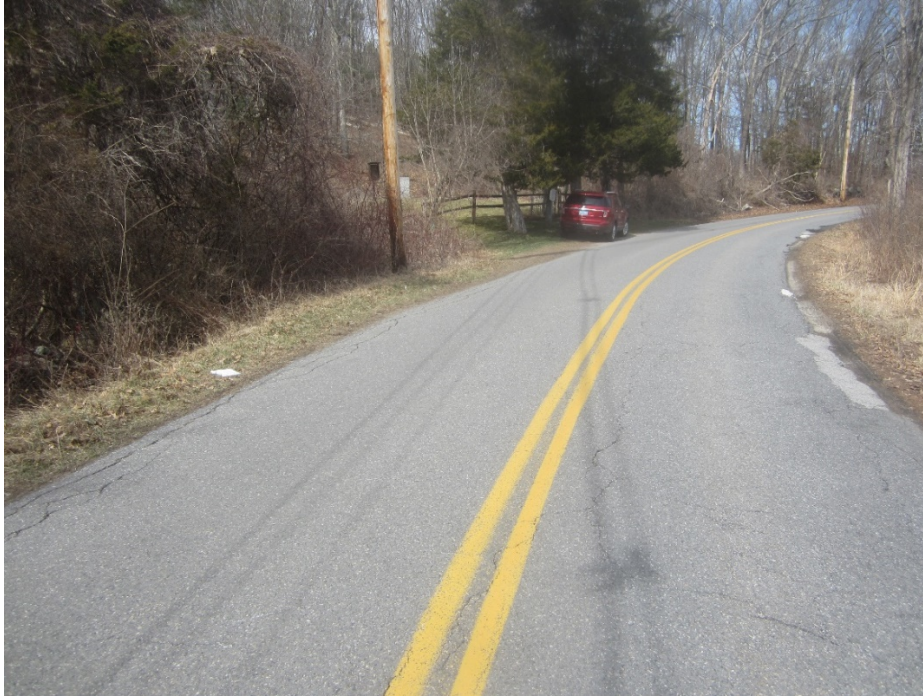
Picture 1 of 2: Culvert inlet is located close to the white clipboard on the grassy shoulder.
