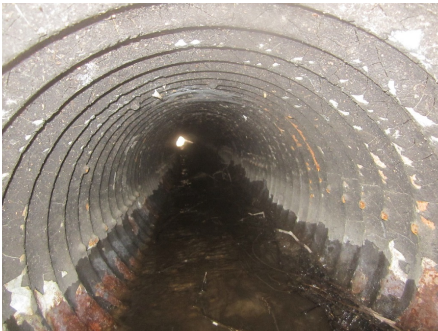
Picture 2 of 2: Corroded corrugated metal pipe.
