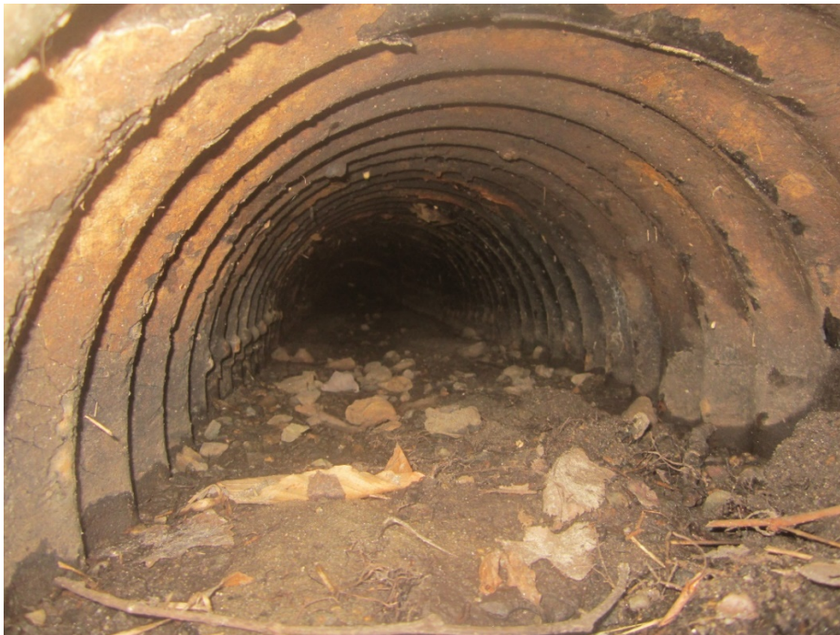
Picture 2 of 2: Corroded and clogged corrugated metal pipe.
