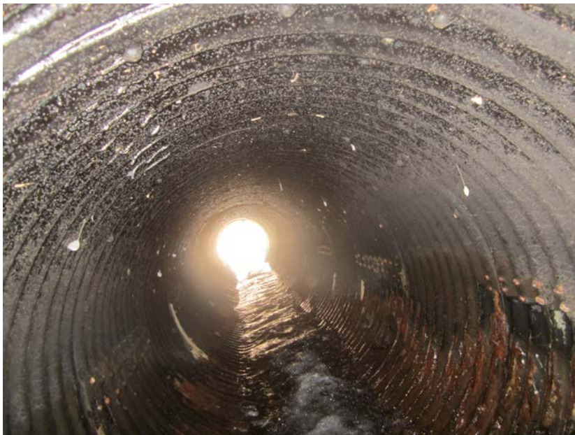
Picture 2 of 2. Corroded corrugated metal pipe.
