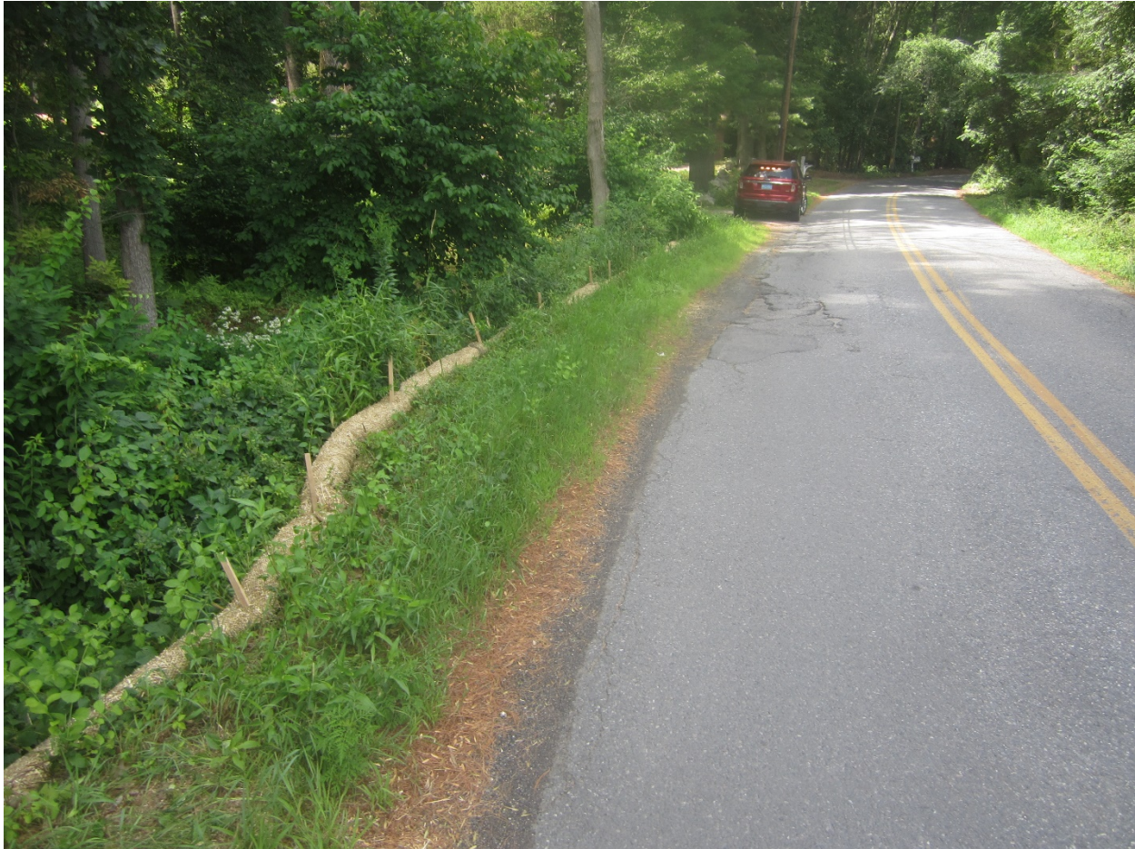
Picture 4: 173 Water Row: Earthen berm on edge of roadway contributes to stormwater ponding and roadway deterioration.
