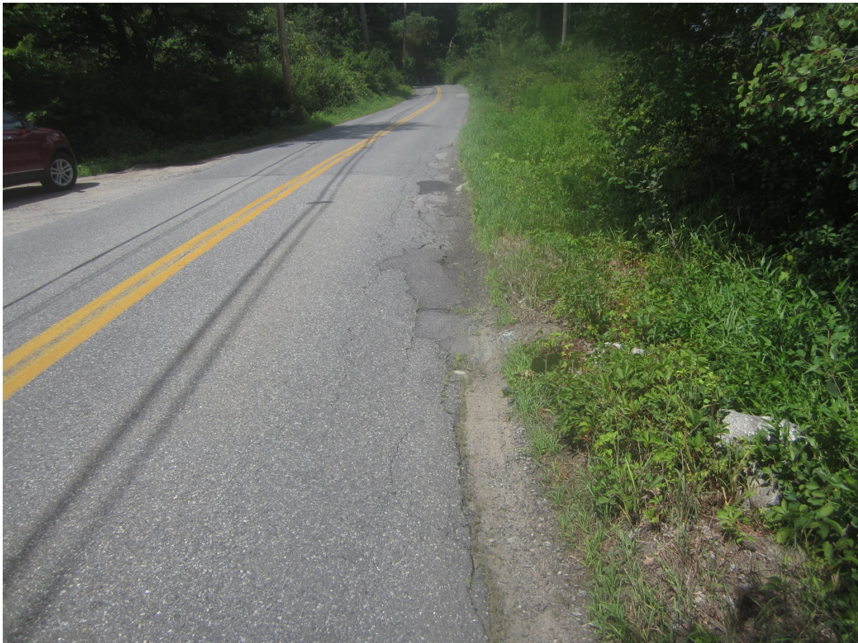
Picture 3: Across from King Philip Woods Parking Area: Low-lying area where ponding stormwater had contributed to roadway deterioration.
