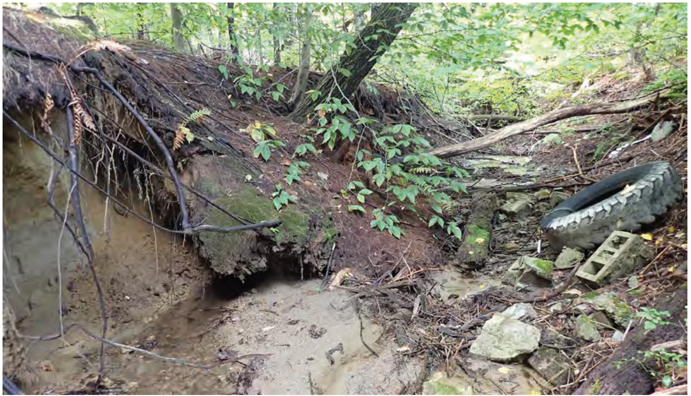
Photo #3: View of another section of the bank where the ground surface has collapsed into the stream due to severe undercutting . Facing south.
