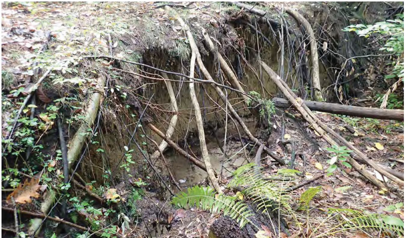
Photo #4: View of section of undercut stream bank. Ground surface collapsing into stream. Facing southeast.
