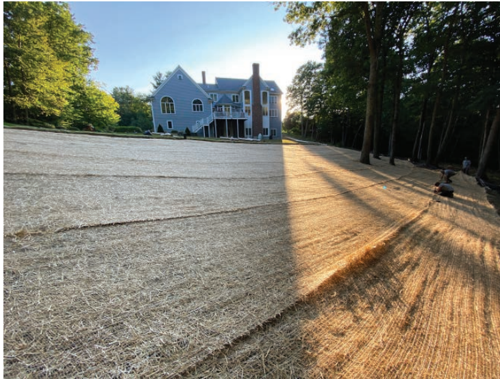
3. Covered exposed loam with straw erosion control blanket: BioNet S75BN and staple into existing slope
