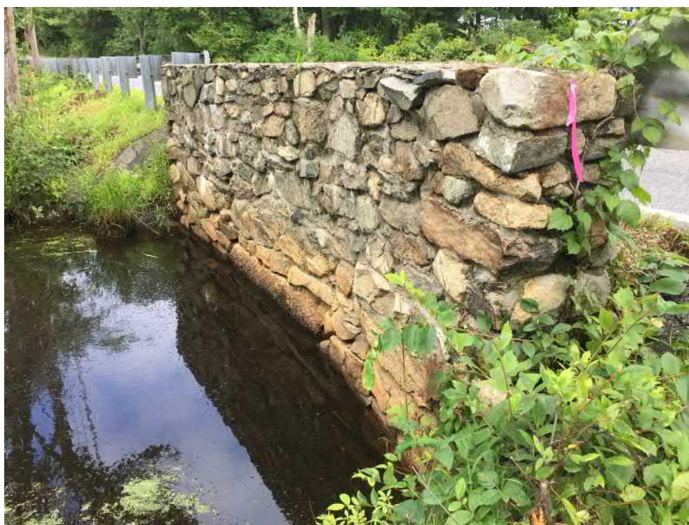
View of the Bank (WF1 Series) at the headwall of Cold Brook—facing northwest
