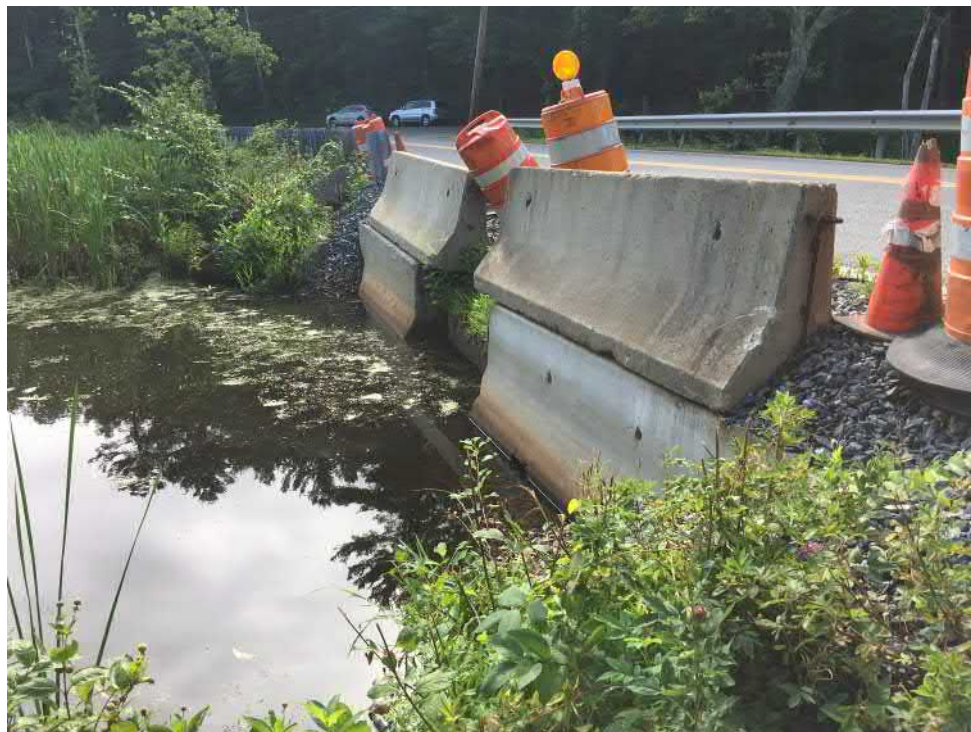
View of the Bank (WF2 Series) at the headwall of Cold Brook—facing southeast
