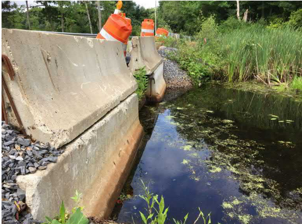
View of the Bank (WF2 Series) at the headwall of Cold Brook—facing west
