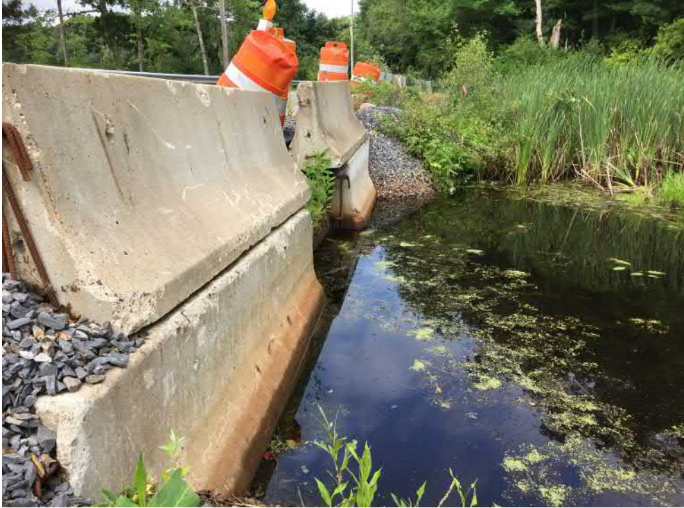
View of the Bank (WF2 Series) at the headwall of Cold Brook—facing west
