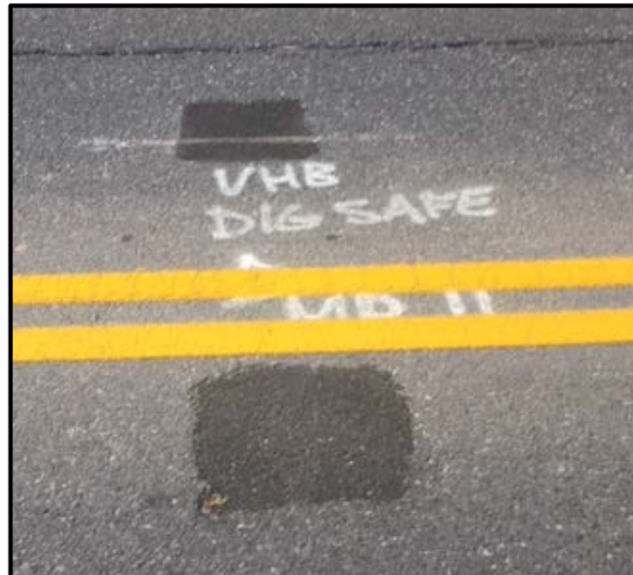
Representative photo showing a test hole after it was excavated and the pavement was repaired
