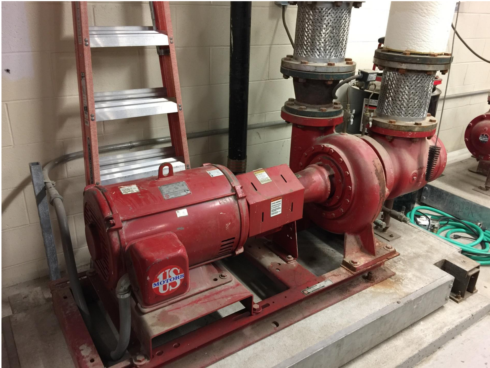
Pump and 40 Horse Power Motor is 18 years old.
