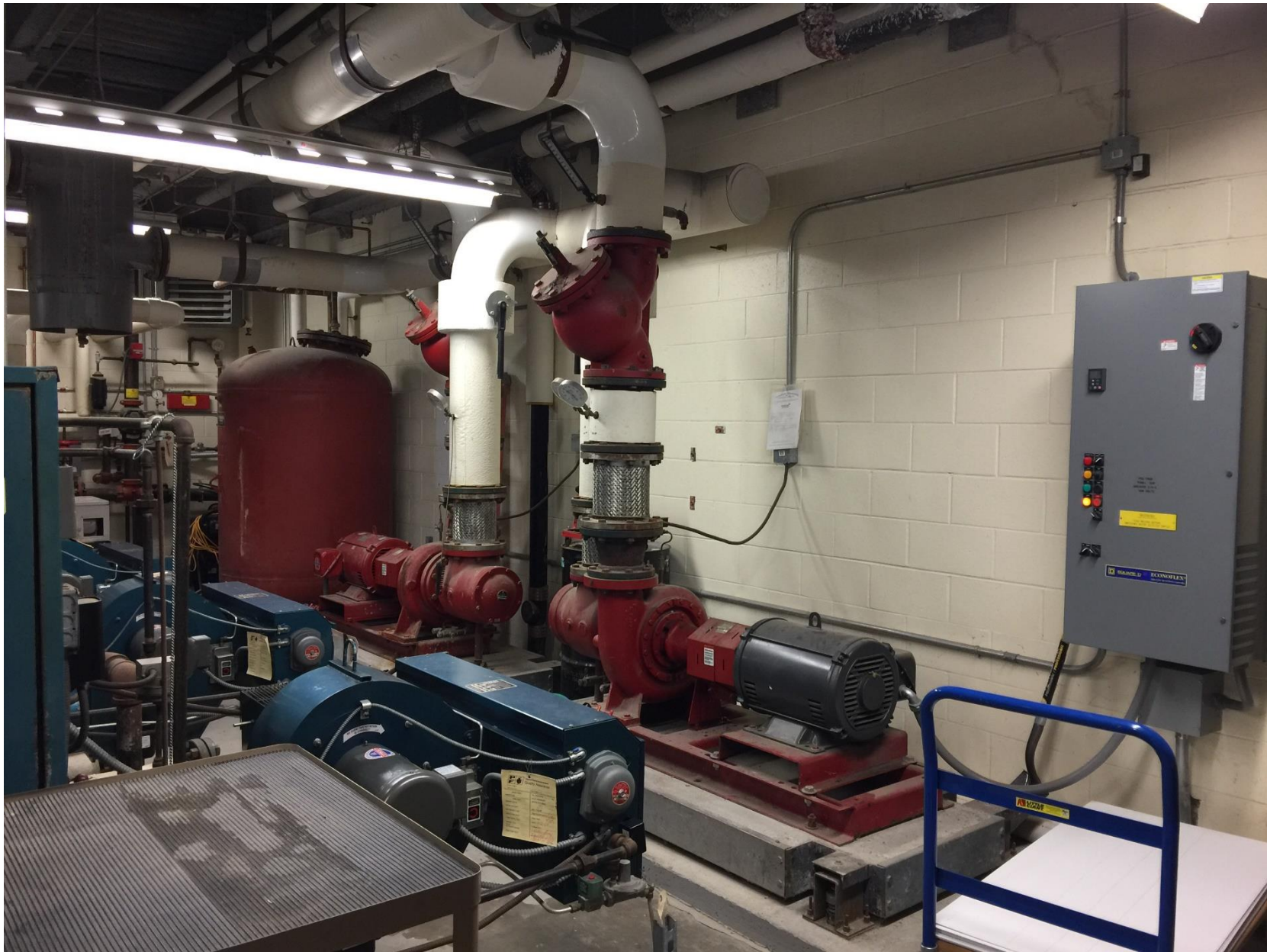
Curtis School Boiler pumps and motors
