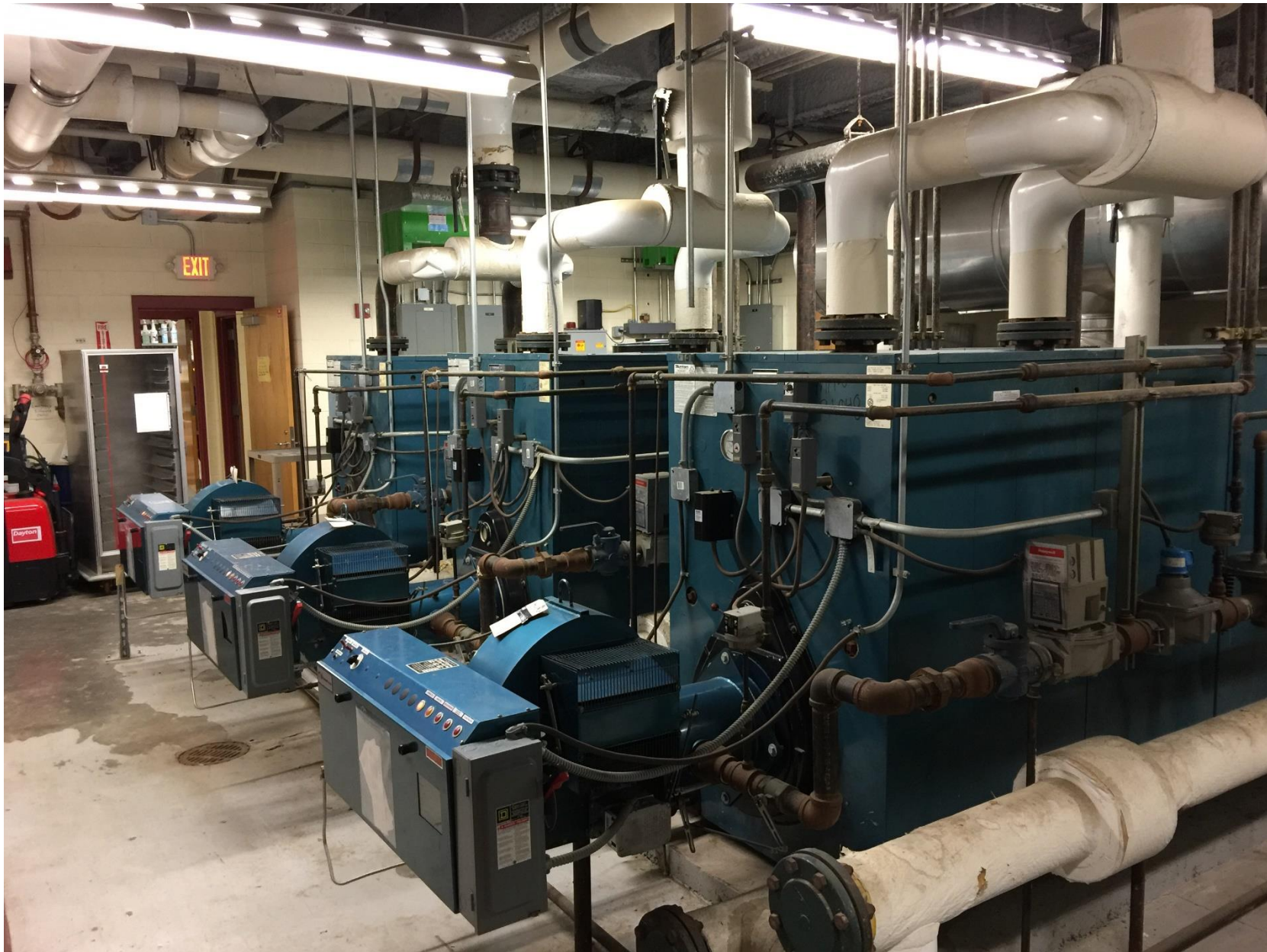
Curtis School Boilers
