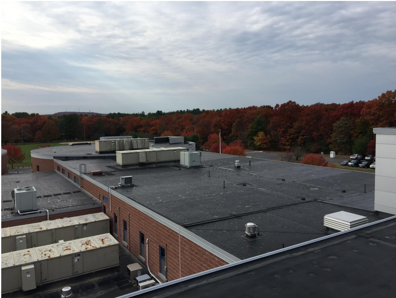
Picture of Curtis roof, showing just some of the two dozen rooftop HVAC appliances.
