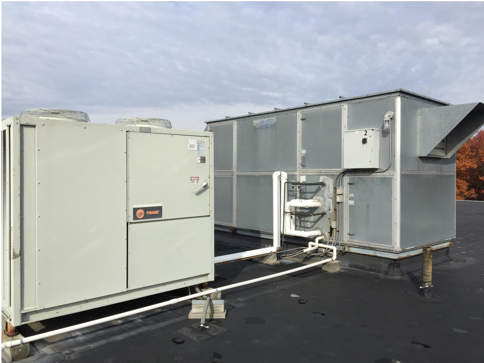
The compressors and air-handling unit for HRU-2
