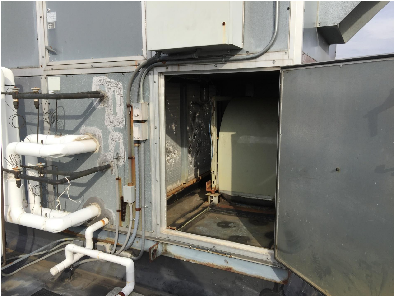
This is the source of leakage and the coils has failed
