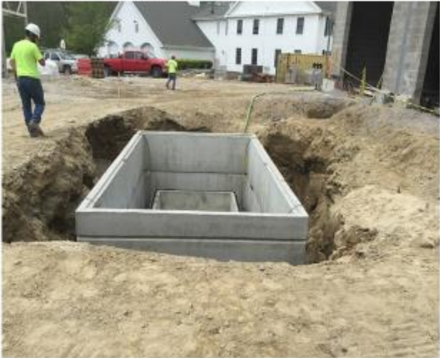
Double Concrete Tanks
