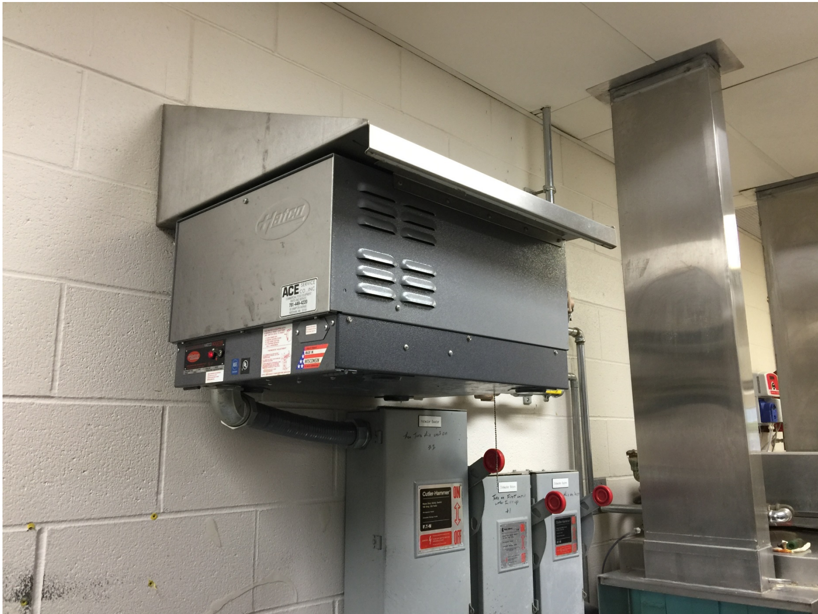
Dishwasher Hot Water Booster
