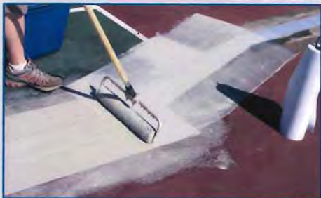
RiteWay Crack Repair System: Laying down micro sealant tape and stress mat.
