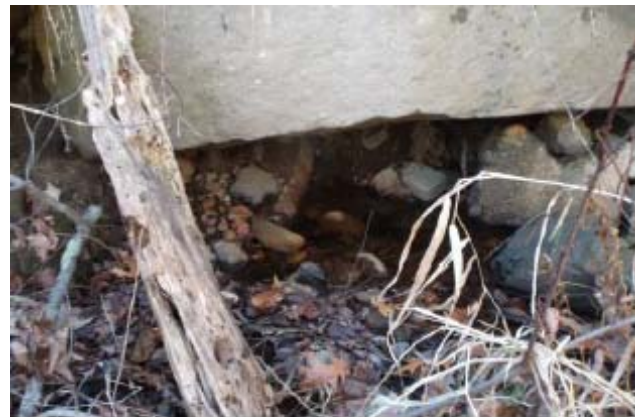
Debris near downstream headwall
