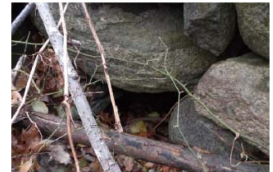
Debris near downstream headwall
