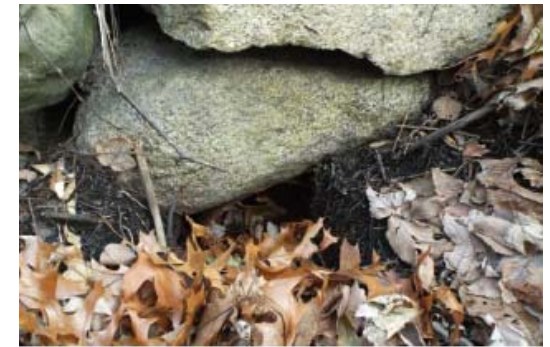
Debris near upstream headwall
