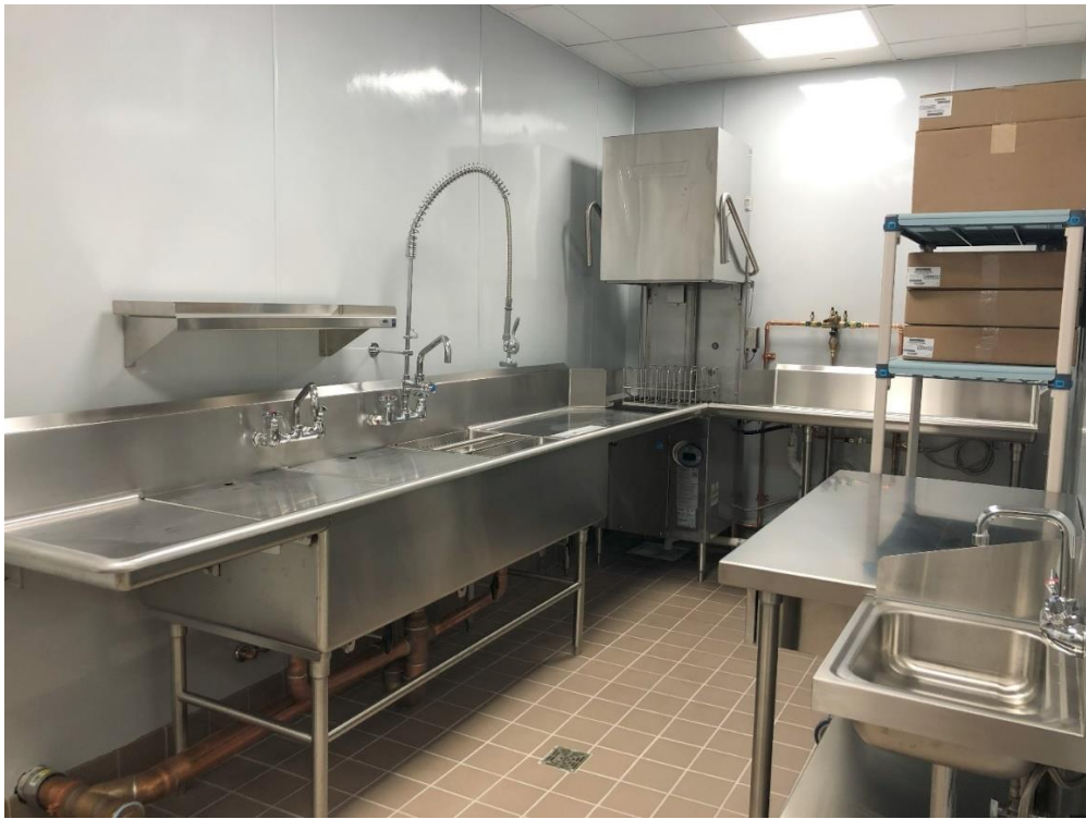
A separate dishwashing station is adjacent to the food prep and cooking area.
