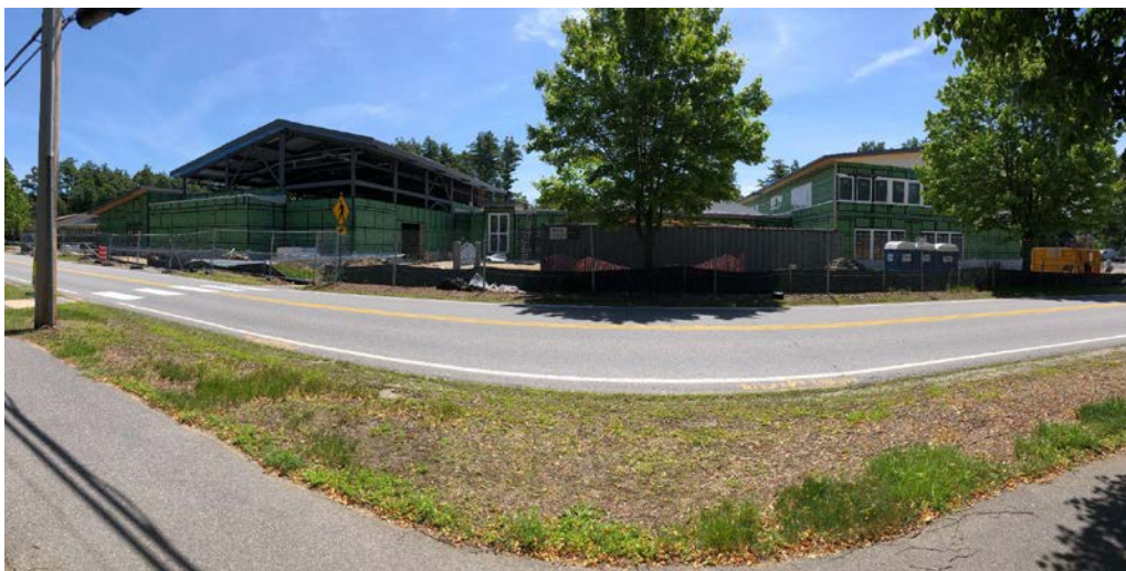
The whole center, with the gym and Park and Rec on the left, SPS and Senior Center on the right, and shared spaces and an outdoor “Commons” lawn in the center.
