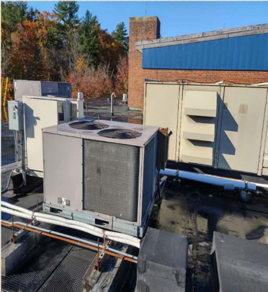
Haynes Library AC Replacement
