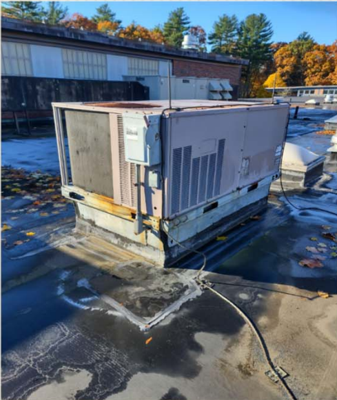
Haynes Admin RTU AC Replacement
