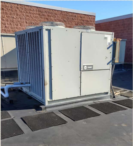
Curtis RTU-12 AC Replacement
