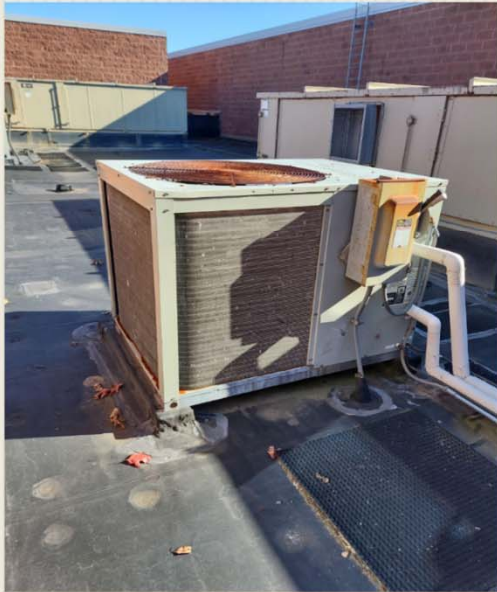
Curtis RTU-9 AC Replacement
