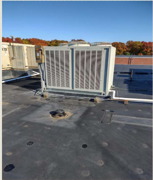
Curtis RTU-7 AC Replacement
