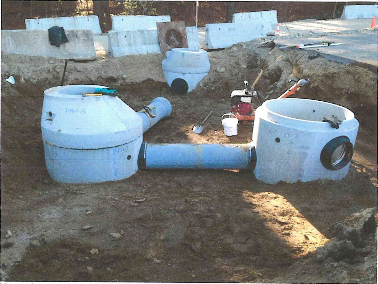
November 20, 2014 – Installation of Drainage Structures (DMH A, CB-1, CB-2) and interconnecting pipe at Musketahquid Drive
